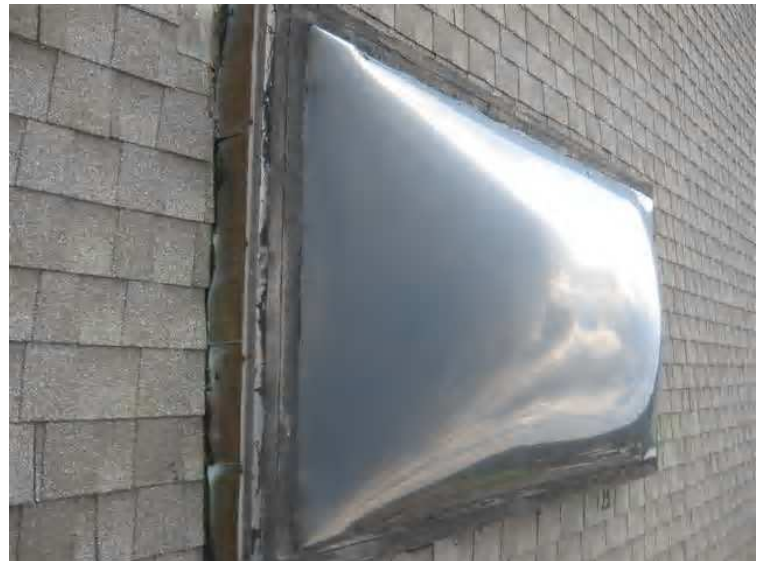
Roof - Both of the roofing skylights [Building B] have been extensively patched with roofing cement, presumably due to previous leakage.
