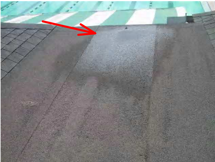
Fitness Center Roof - Shows low spot where water is pooling
