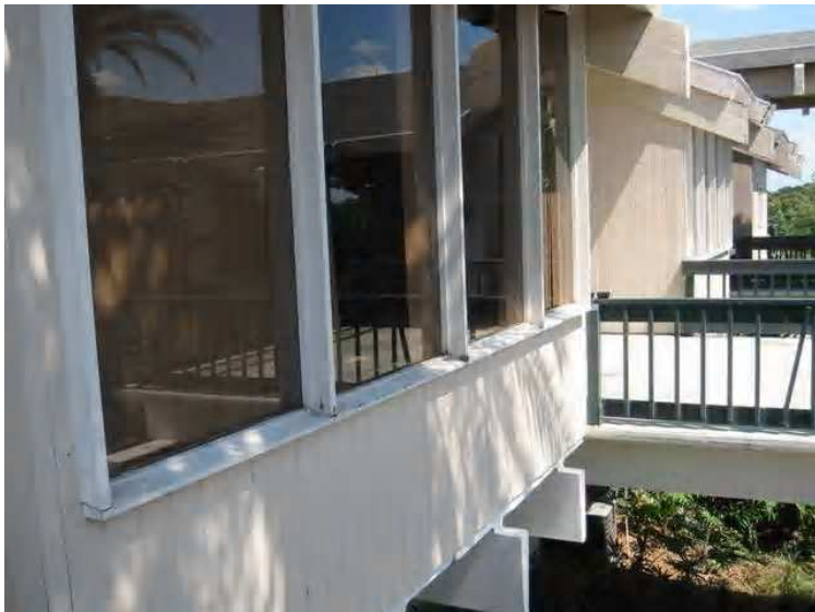
This image depicts significant rot and moisture damage to a window on the south side of building B. As previously mentioned we recommend further evaluation of all window frames on the structure.
