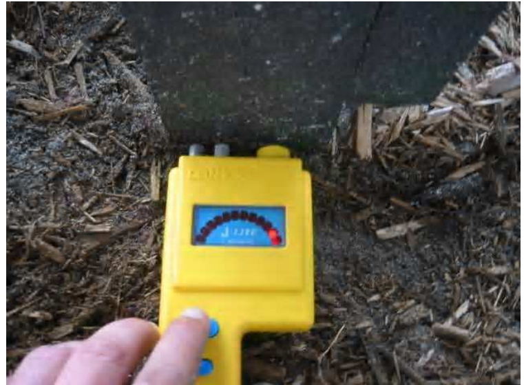
This image shows elevated moisture readings at the base of one of the support columns supporting the wooden stairs coming off the deck on the south side of building B. [see diagram 1 for location off BD3]
