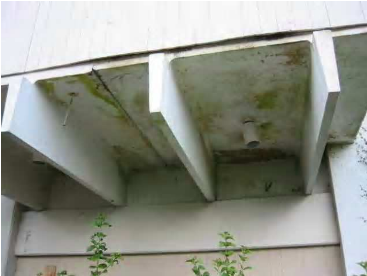
Structure - Cantilevered section of the second-floor kitchen in Building B. Condensation from the refrigeration units has been allowed to permeate this overhang resulting in significant rusting of the structural embedded steel, damage to the walls framing and siding and considerable mold, and bacterial growth on the underside of the floor structure.
