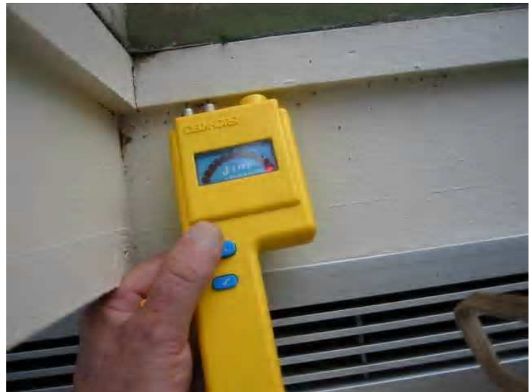
Picture showing elevated moisture readings on an interior frame in the 2nd floor members dining room in building A. this frame is showing moisture in excess of 30%.
