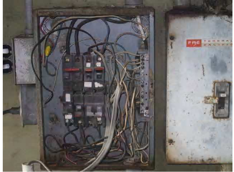
Pump House - The electrical system is designed as NEMA 1 which is indoor only, all electrical equipment has been exposed to the weather over a long period of time and should be abandoned and replaced.
