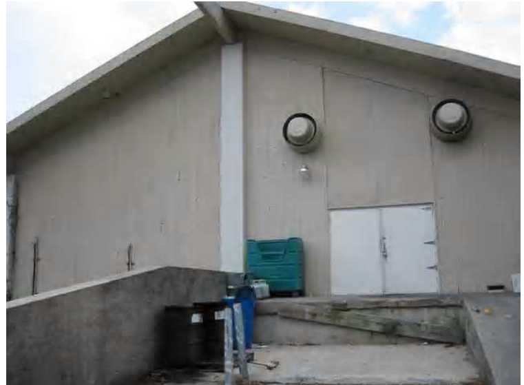
Building B. 2nd floor loading dock, the siding in this area is rotten due to moisture intrusion in the attic space from improper flashing and caulking of the siding materials. We recommend further evaluation of the sill plate, as it could not be viewed at the time of inspection.
