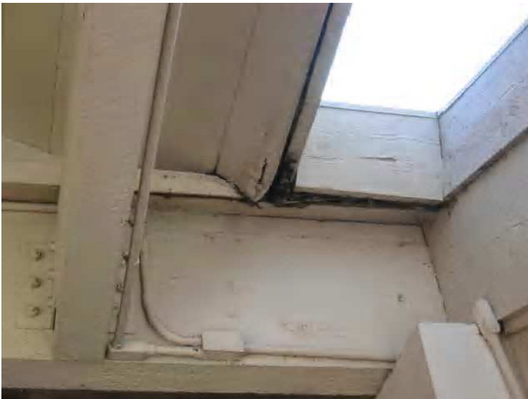
Roof - This picture is of the soffit and fascia area under the connection of the breezeway and building A. extensive rot and decay is clearly visible. And we recommend further evaluation of these areas by a licensed roofing contractor at the very minimum.
