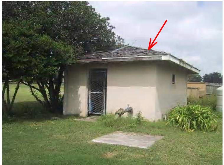
Pump House - Note the roof which is in eminent danger of failure and collapse.
