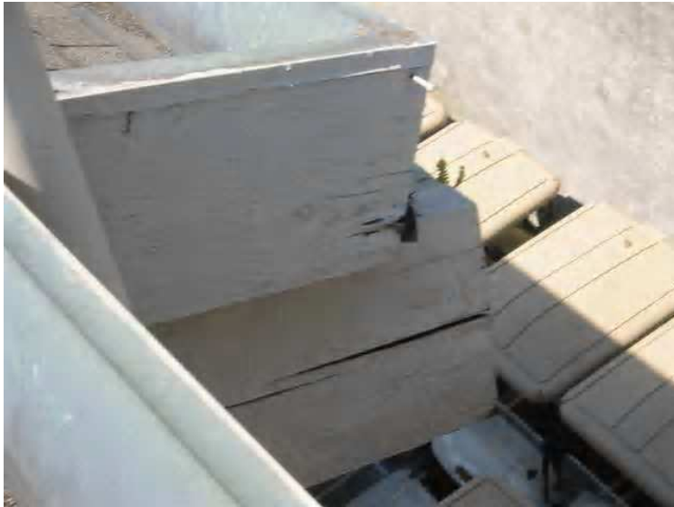
Roof - This image [taken on the south side of building B.] again shows damage to the fascia, soffit and roof rafter, and requires further evaluation.
