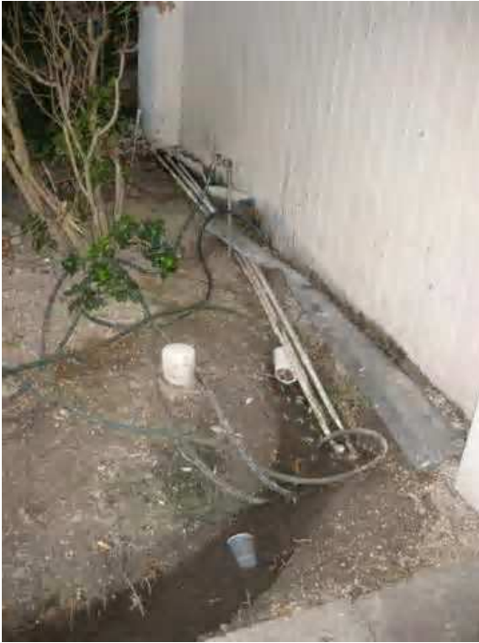
South west side of building B. and shows damaged condensation lines. Due to inadequate drainage all of this condensate is being retained directly against the structure's siding and sill plate in this area.
