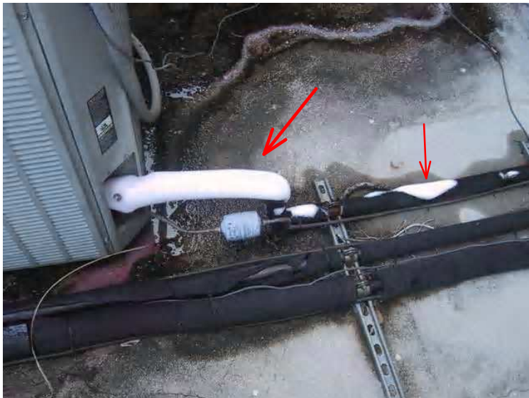
Split-system A/C condenser units showing frozen refrigerant lines this is usually a sign of low refrigerant in the system.
