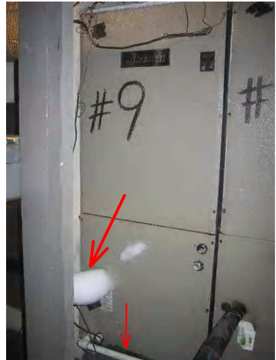
Typical air handler - Air handler units and associated ductwork are mostly original to the building and show signs of mold contamination. Note the frozen refrigerant lines.
