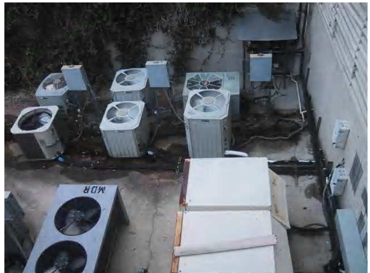
HVAC Condenser's - Split-system A/C condenser units in various stages of deferred maintenance. Note: leaking condensation, frozen refrigerant lines, mold like substances.
