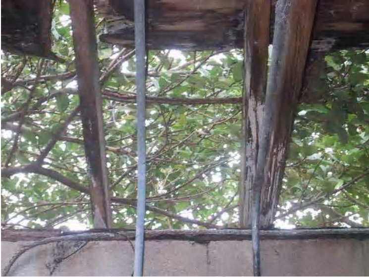
Pump House - The roof is no longer providing protection to the interior of this building.
