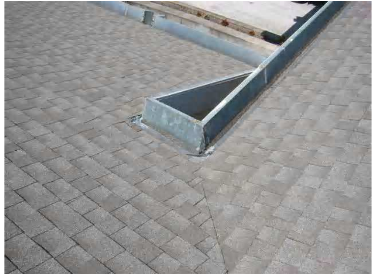
Roof - This image shows the flashing detail at the connection of the entryway roof to building A. it appears that all of these type interfaces between the roofing junctions have failed allowing moisture entry into the roofing fascias, soffits and sheathing.
