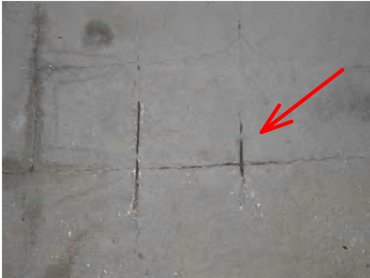
Structure - Welded mesh embedded into the poured concrete walkway on the breezeways between buildings was left to close to the surface, see full report.
