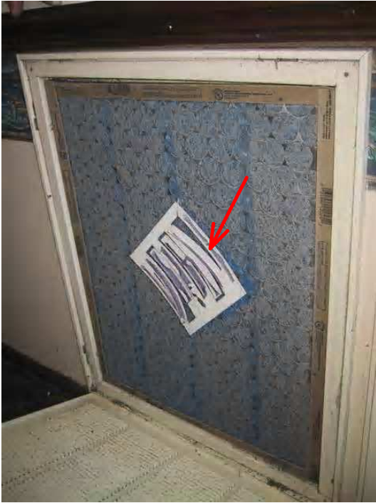
Typical HVAC return filter - Note the air freshener attached to the filter used mask the mold odor. The entire HVAC registers and ductwork will need to be professionally cleaned.
