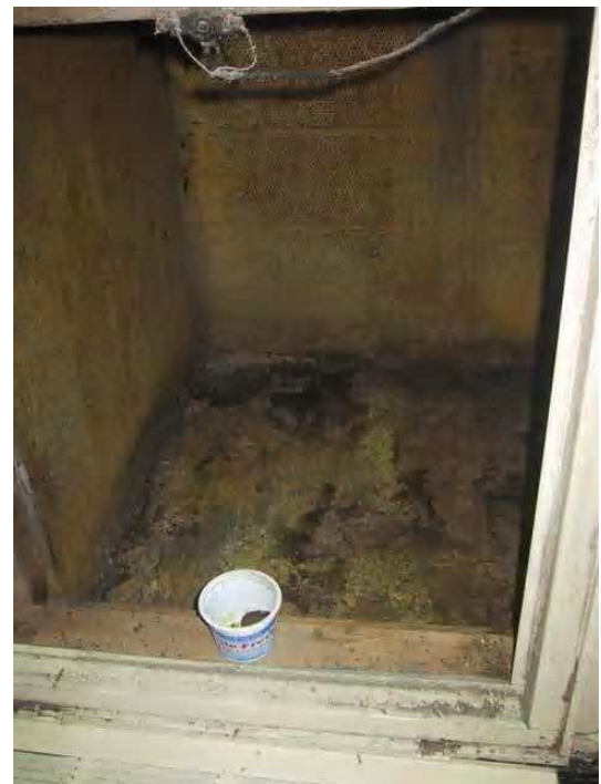
Typical HVAC return duct - Note the dirt and probable mold-like substances growing. The entire HVAC registers and ductwork will need to be professionally cleaned.
