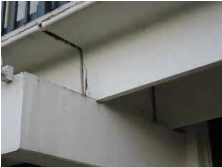
Structure - The deck area on the eastern end of Building B [BD2 diagram 1]. Damage to both portions of the bearing surface has led to expansion of the structural steel, resulting in spalling of both the grade beam and the deck support.
