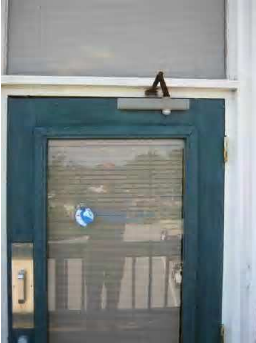
This door leads from the offices in Building A to the exterior deck [AD1 on diagram 1] there is evidence of moisture intrusion into the door framing which forced the door & jamb out of plumb.
