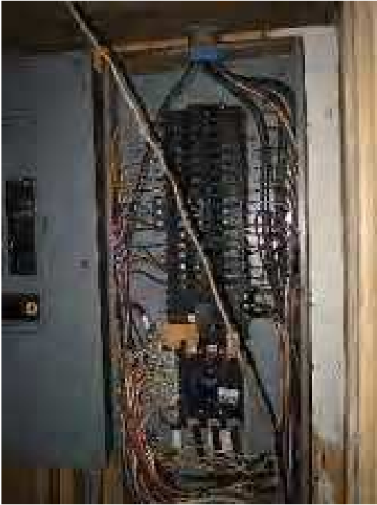
Maintenance Buildings - The electrical service in this building is in an unsafe condition, see full report.
