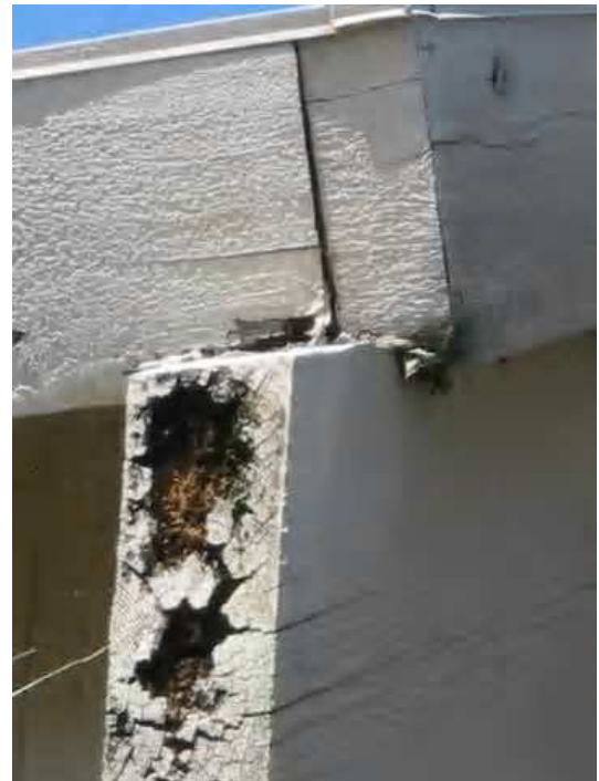
Roof - Leaking through the flashings resulted in rot to the Fascia, soffits and the exposed end of the rafter tail, see full report.
