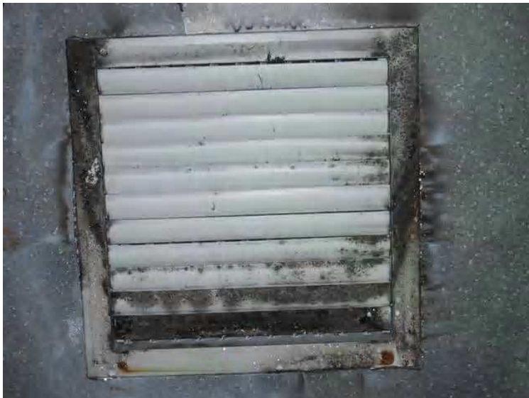
Typical HVAC register - Note the dirty discharge and probable mold-like substances growing. The entire HVAC registers and ductwork will need to be professionally cleaned.
