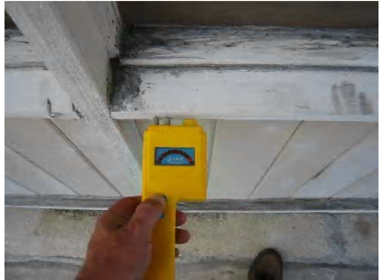
2nd floor office windows as seen from deck [AD1] elevated moisture readings only confirm the visual evidence of rot in the window frame, this is typical of the window elements on both buildings.
