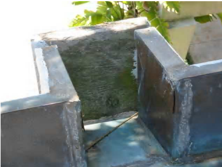
Roof - Copper scupper detail on the south side of building A. Many areas of the roof the flashings were disturbed by recovering the roof and the joints were re-adhered using roofing cement rather than being re-soldered, see full report.
