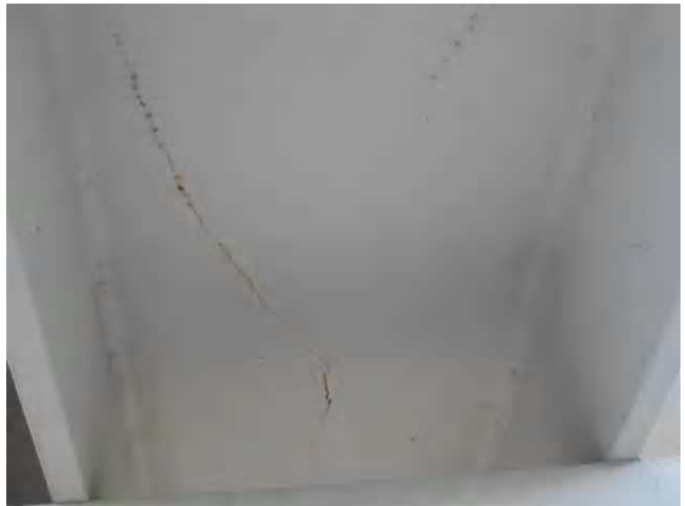
Structure - Deck depicted immediately above [BD2 on diagram 1] the line that can be seen on the underside of the deck is of a crack or fissure presumably running right through the deck, as it is showing signs of moisture intrusion, leaving rust stains along the crack.
