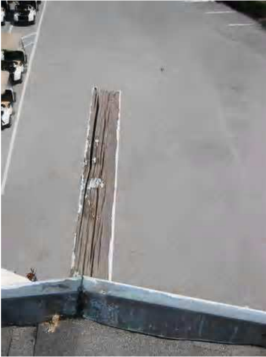
Roof - Projection area of the ridge beam on the eastern end of Building A. this damage is typical of all the exposed timbers projecting past the gable ends. The damage has been brought about by lack of maintenance [particularly lack of painting and caulking on a regular basis.
