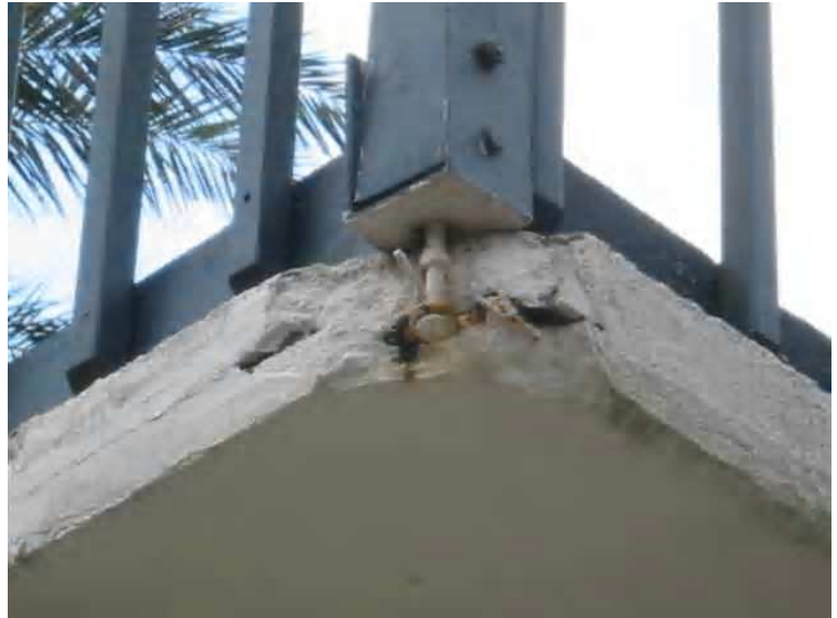
Structure - moisture intrusion has affected the ferrous metal fastenings of the safety railing, a metal retaining bolt has expanded due to rust, see full report.
