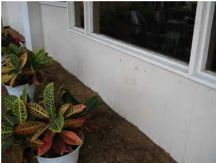
This image [typical of all areas] is on the north east side of building B. here the grade level is in contact with the siding leading to elevated moisture levels and rot damage [all wood siding materials should be a min of 6 inches above grade]
