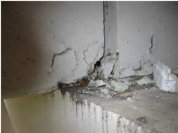
Structure - Failing deck bearing to grade beam connection [BD4 diagram 1] this damage is typical of all of the bearing connectors that should be supporting the live and dead loads associated with this structure.
