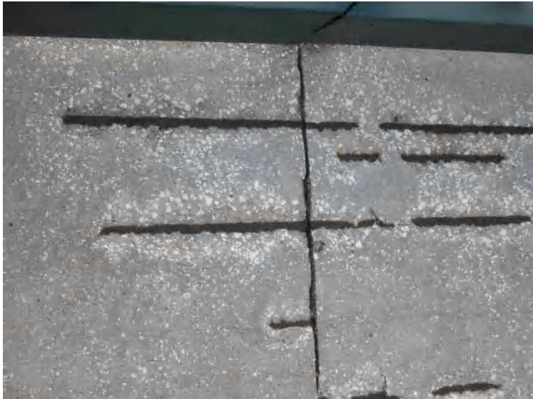
Structure - Building. B. [BD3 on diagram 1] the structural steel ties between structural elements were installed to closely to the surface, erosion and wear have left these exposed to the elements. This again is a structural problem, as the steel serves to tie the elements together.
