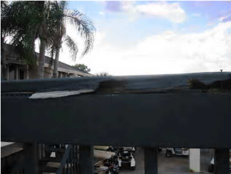
Handrail on east side of deck [BD4 see diagram 1] this handrail is typical of all inspected on the property as it has been damaged by either rot or termite activity, we recommend repairs or replacement as needed.
