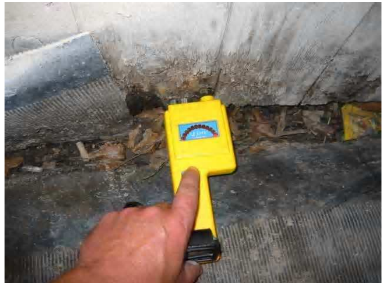
In this image [taken on the south west corner of building A.] the moisture meter is showing readings exceeding 30%, moisture levels this high cause the siding materials to rot.
