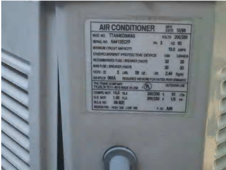
Typical AC Compressor manufacturers plate: The compressors have an average age of 8 years and an average cooling capacity of 4-tons.
