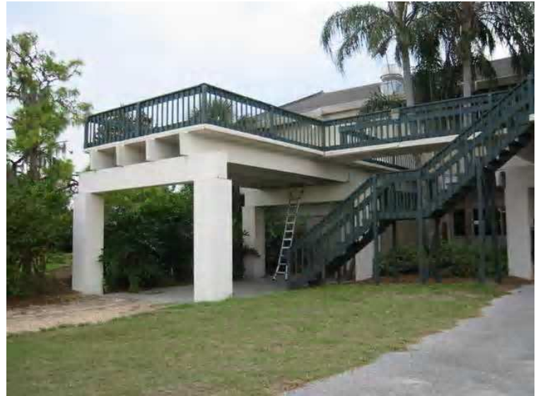
Structure - [BD4 diagram 1] it is this deck that poses the largest structural problem at this time,. There is considerable damage due to corrosion and spalling around the bearing surfaces. It also appears that there is possibly some rotation of the grade beam supporting the end of this deck.
