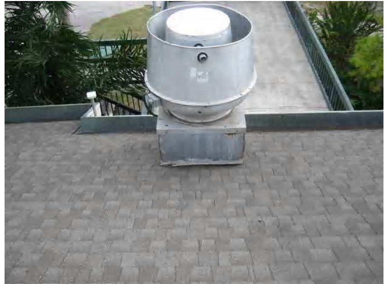
Roof - Pictured to the right is the vent for the kitchen extractor fans on the south west side of building B. This vent has defective flashings allowing moisture to enter the building [see interiors report]
