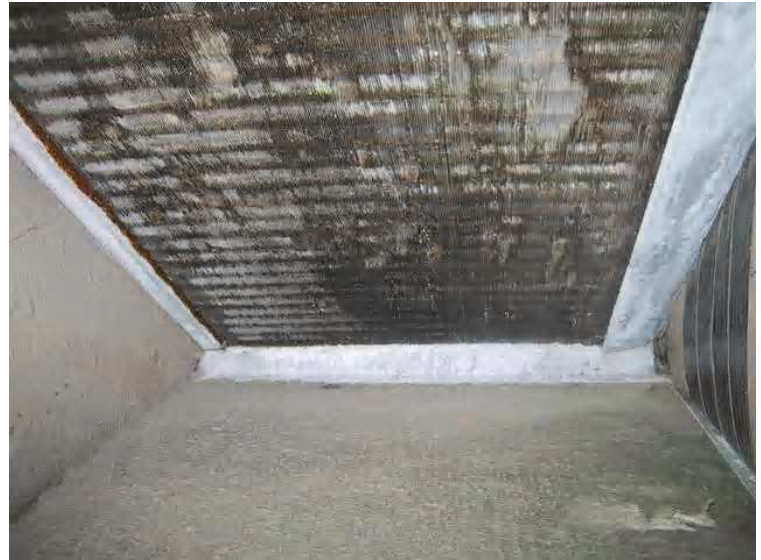
Typical HVAC cooling coil - Note dirt and clogged cooling fins. The entire HVAC registers and ductwork will need to be professionally cleaned.
