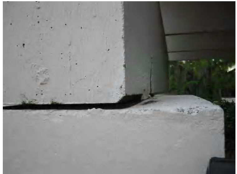
Structure - The picture appears to show signs of rotation of the grade beam supporting the extreme edge of the second-story deck [BD4 on diagram 1]
