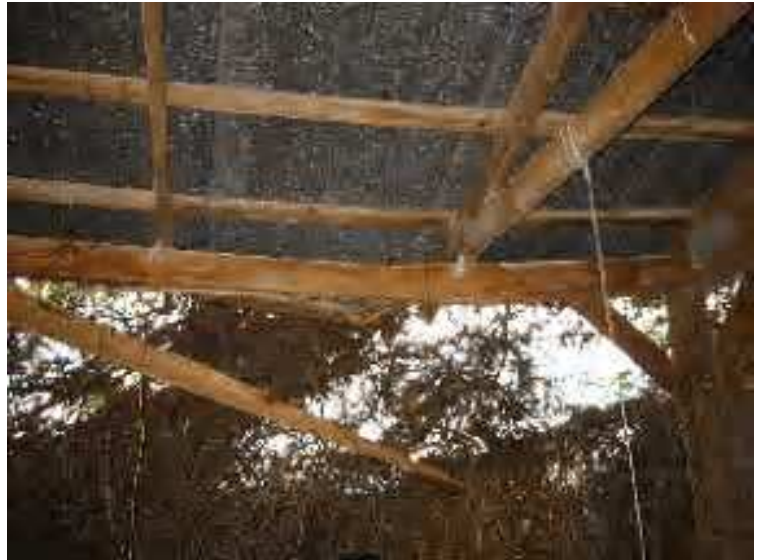
Maintenance Buildings - The cart storage barn roof is in particularly poor shape possibly from previous storm damage, see full report.
