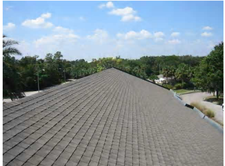
Roof - This picture shows the roof covering over Building A. [see Diagram 1] the coverings and sheathing show signs of settlement on the Western end of the structure. Possibly due to rot as noted in the exposed ends of the rafter framing.
