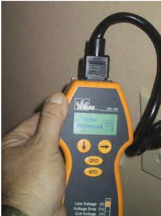
Typical non-grounded receptacle. This condition is most likely related to the damaged conduits in the electrical riser system, further evaluation by a licensed electrician required.
